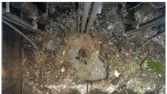
Pictured: Debris crust that had formed at the top of the wet well.
