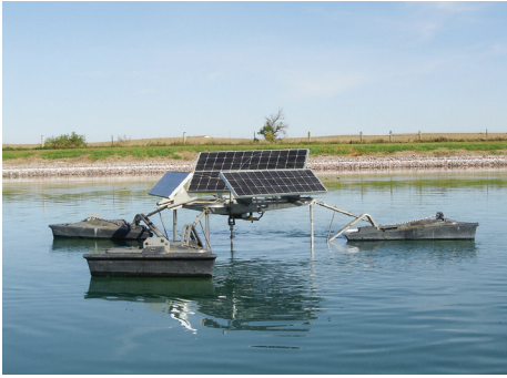
SolarBee mixers circulate and oxygenate the top half of the wastewater treatment pond, "capping" and preventing odors from escaping to the atmosphere.
