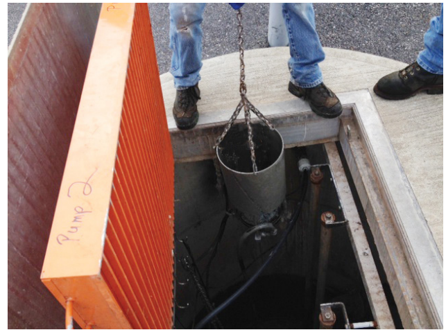
Installing the AP500
