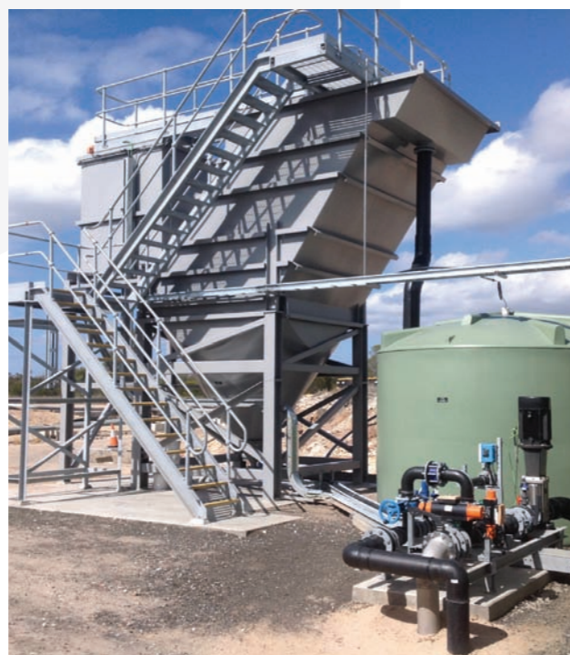
Stormwater Treatment for Reuse - 75 m 3 /hr - Clarifier - QLD
