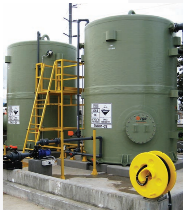
Bulk Chemical Storage & Dosing System - 2 x 25 m 3 capacity - TAS
