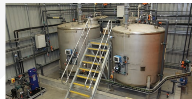
Contaminated Ground Water Treatment Plant - 60 m 3 /d - Fenton Process - VIC
