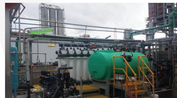
Backwash Wastewater Treatment Plant - 1 ML/d - UF - NSW
