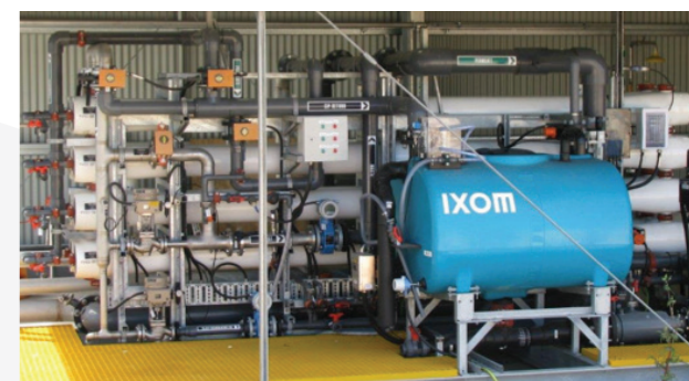
Bore Water Treatment Plant for Boiler Feed Water - 0.9 ML/d - RO - QLD
