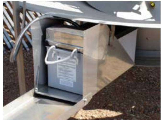
Battery Lid Down, Battery Lead Out
