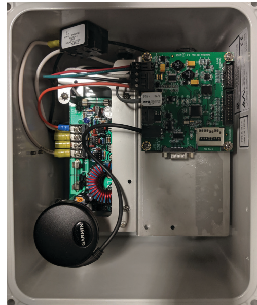
Figure 2: SB A-Series Control Panel, Internal
