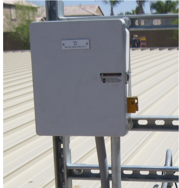
Electronic Control Box of an Underground Reservoir
