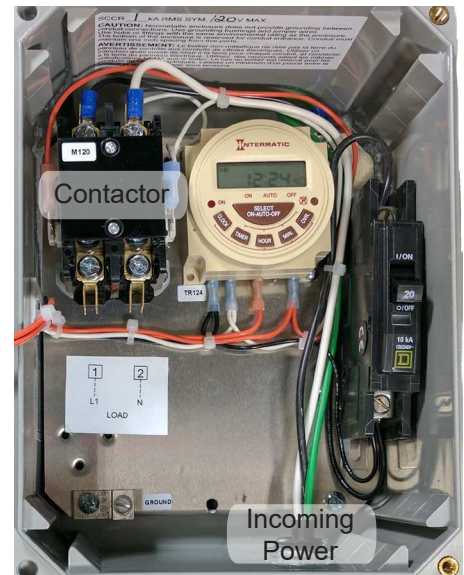
Figure 2: Disconnect Control Panel
