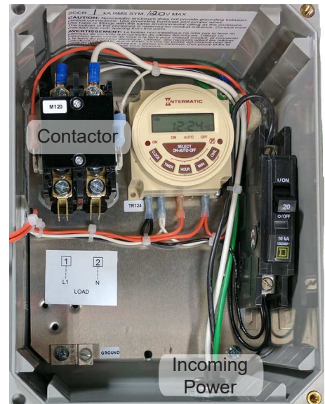
Figure 2: Disconnect Control Panel
