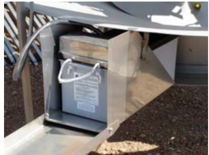
Battery Lid Down, Battery Lead Out
