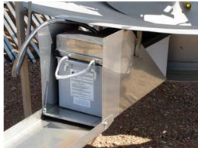
Battery Lid Down, Battery Lead Out
