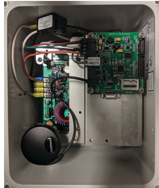
Figure 2: SB A-Series Control Panel, Internal
