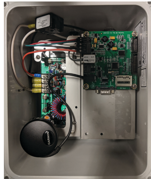
Figure 2: SB A-Series Control Panel, Internal
