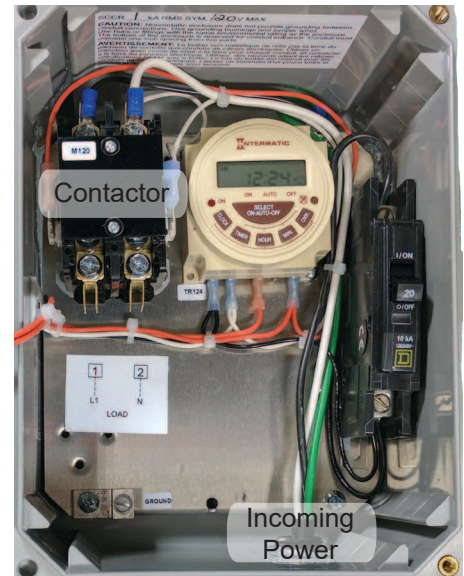
Figure 2: Disconnect Control Panel
