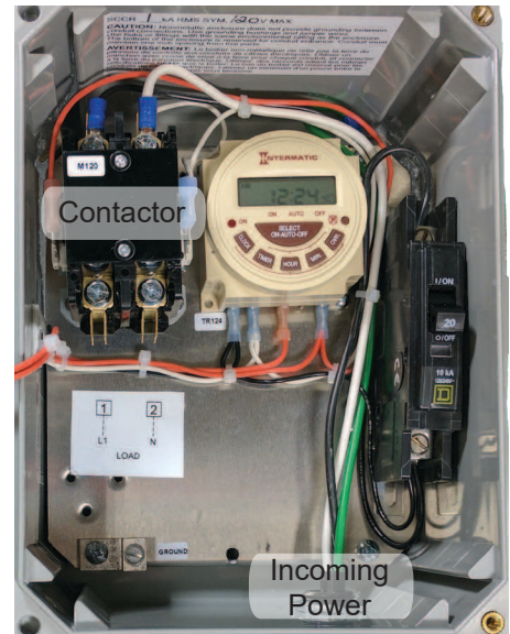
Figure 2: Disconnect Control Panel
