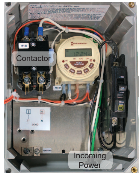
Figure 2: Disconnect Control Panel
