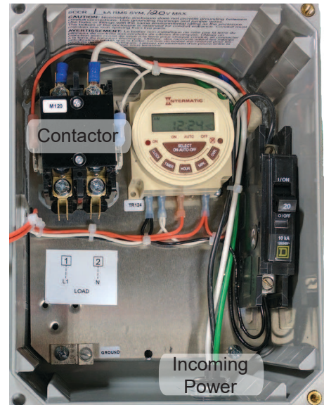
Figure 2: Disconnect Control Panel
