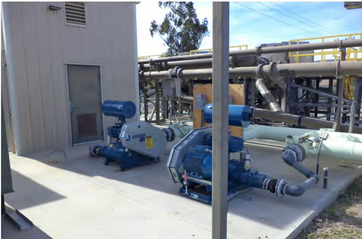
After – Replaced (3) 75hp air units with (2) 25hp air units
