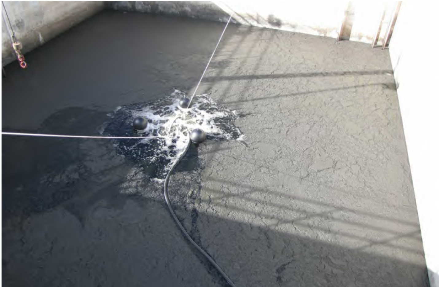
AP7000F Floating Style Mixer in basin, recently started
